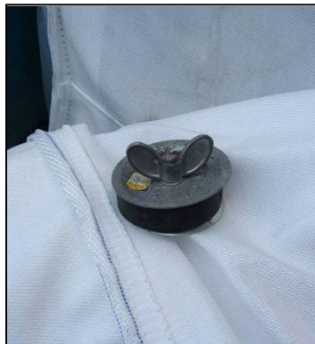
Plug to Isolate Drainage Line
