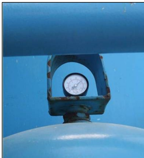
Blast Pot Pressure Gauge
