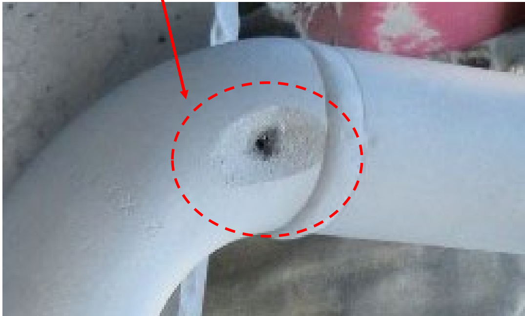
Corrosion blister of a large size Closed drain, small diameter, thin wall
